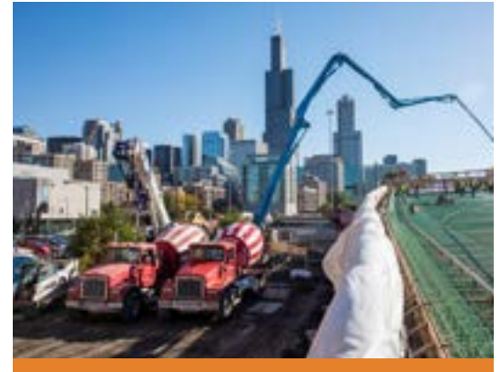
Ozinga Ready Mix has been producing CO 2 mineralized concrete via CarbonCure since 2016.
